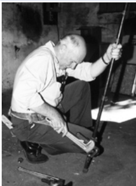
Doré Westra fitting a pipe in a client's basement, circa 1990. During the 2008 Resourceful Homeowners Celebration, Dave Jacobs honored Doré Westra for his three decades of helping lower-income families in Kent County. The story at right is an excerpt from Dave's tribute.
